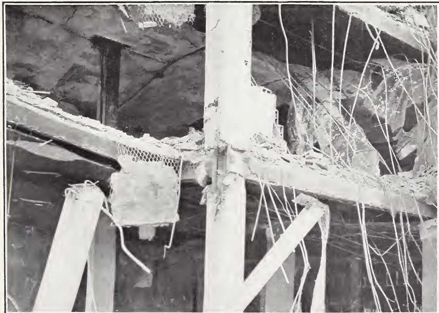
B. DAMAGE SAID TO HAVE BEEN CAUSED BY DYNAMITE, RIALTO BUILDING.
